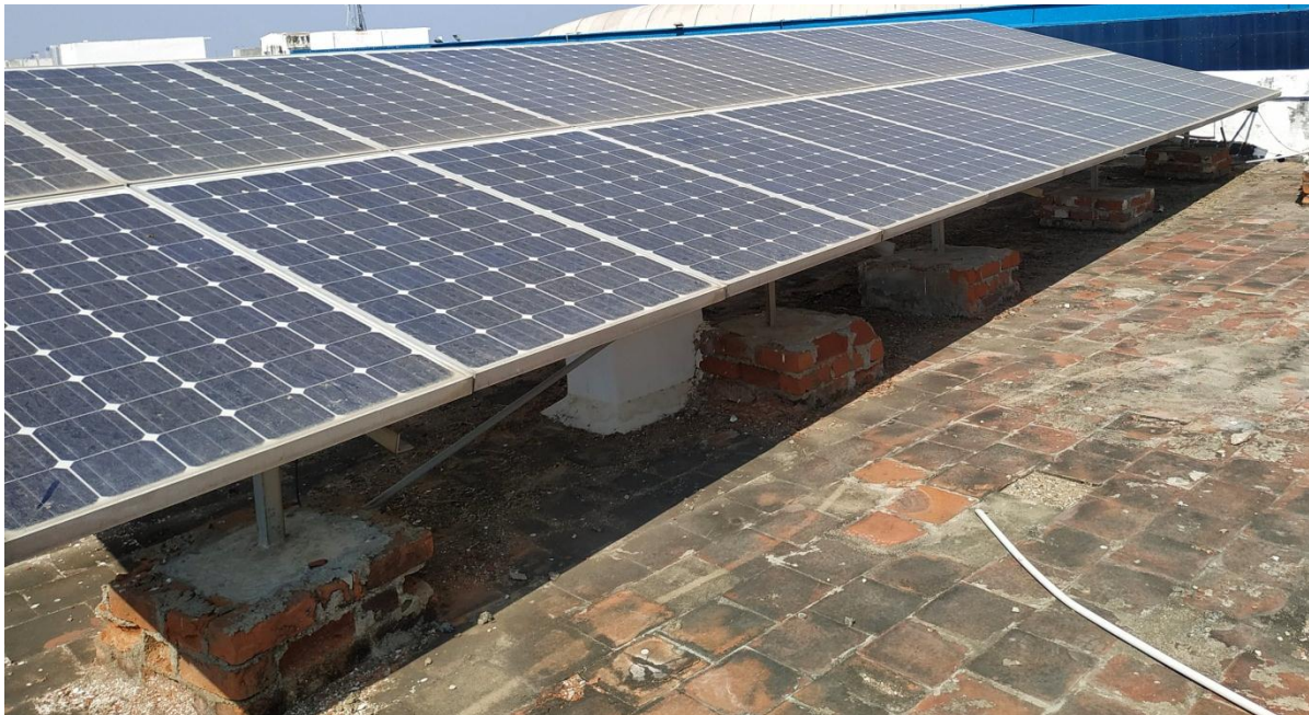
6kW capacity installed in the Class Room Block
