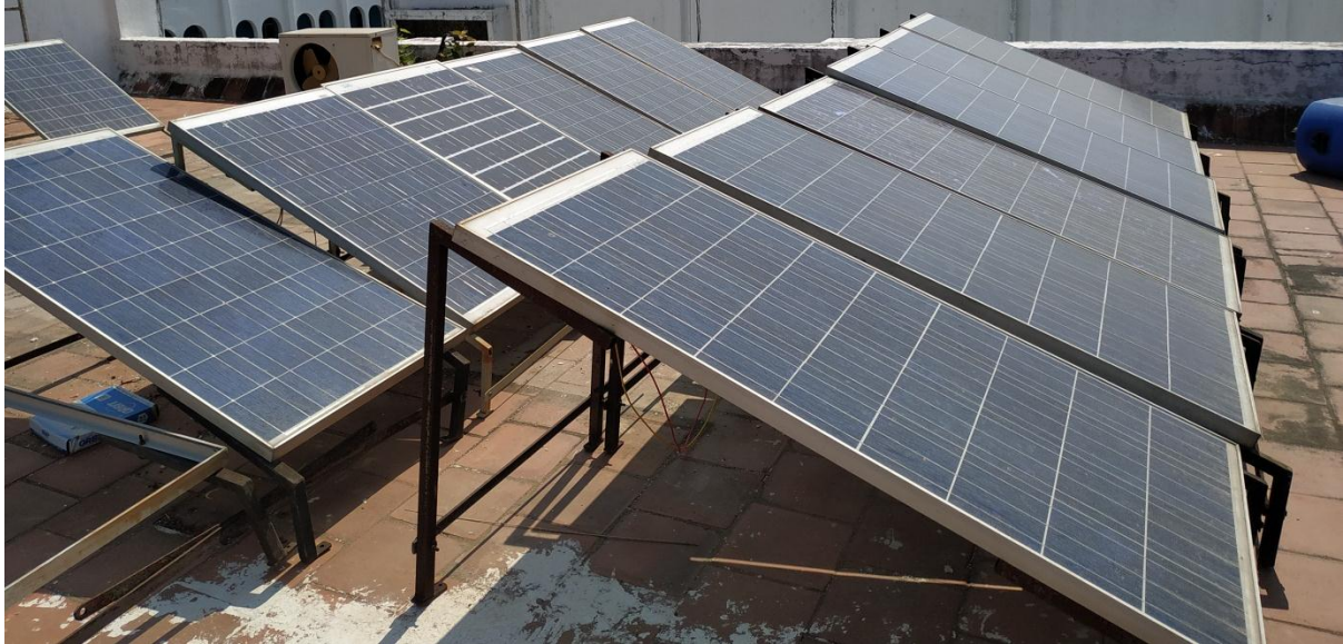
5kW capacity installed in the Laboratory Block
